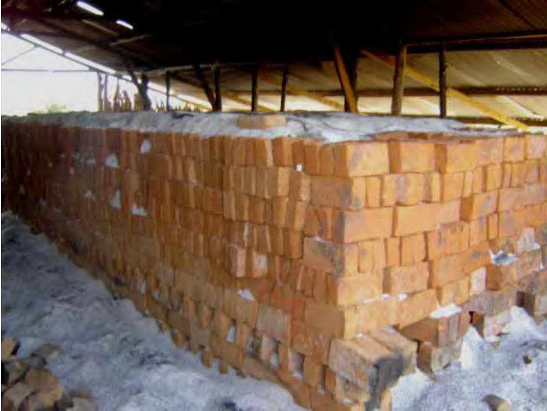
“fired bricks under the shed with clamp kiln. It needs a shed during rainy seasons.”
