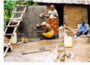
UGANDA, Kyotera Construction of a Rain Water Harvesting Tank by women's group for an old village. This will provide clean water close to her home.
