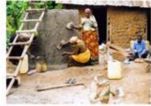
Kyotera, UGANDA Construction of a Rain Water Harvesting Tank by women's group for an old widow. This will provide clean water close to her home.
