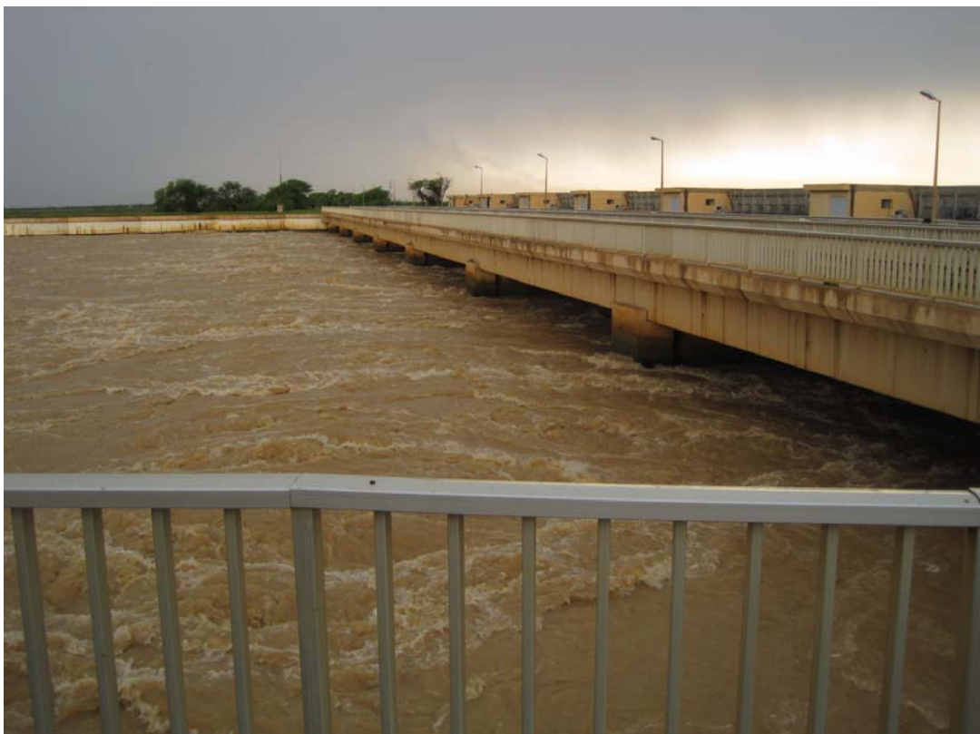
Photo 6: The downstream side of the Dama dam. At the time of the visit the discharge was said to be 1600 m 3 /s.
