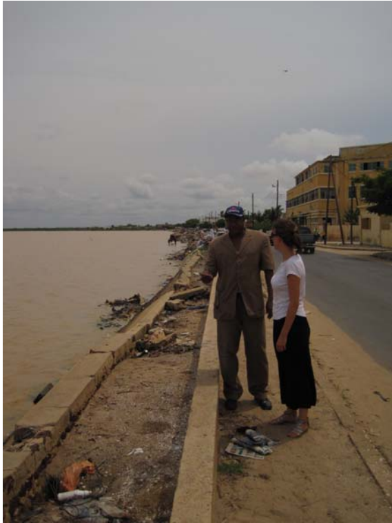
Photo 1: Road along the northern part of Sor (named Boulevard El Hadj Momar Sourang). Poor water drainage from the road to the estuary. Small scattered damages to the wall.
