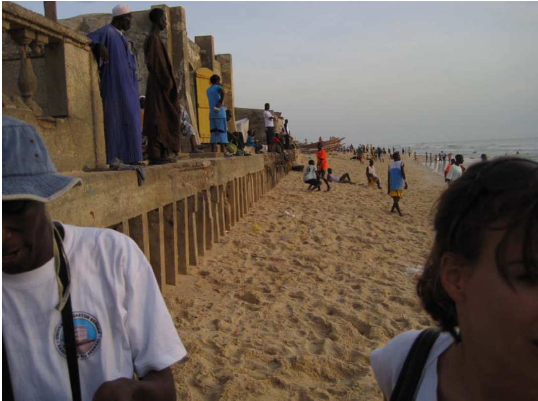
Photo 19: Seawall at Ndar Toute looking southwards. Narrow beach which disappears at high waters (waves breaking on the seawall causing locally some damage). Wall was said to be part of a boulevard built in colonial times (at least a century ago)
